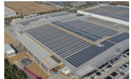
Solar power generation system installed on the rooftop of a plant in China
