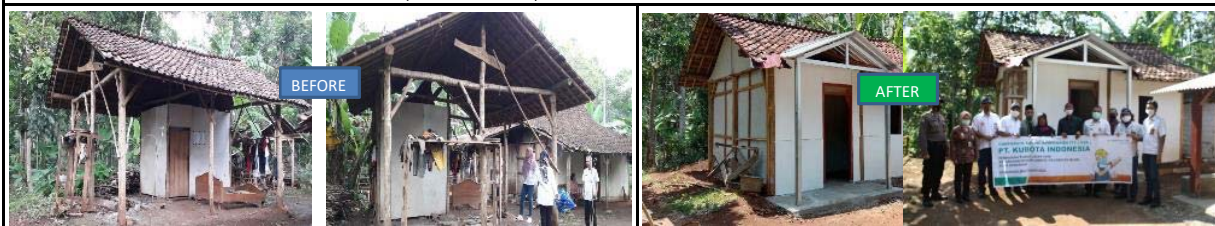
3. House of Mr. NGATIRIN (RT 09 / RW 01) – DS. WONOPLUMBON – KEC. MIJEN – KOTA SEMARANG
