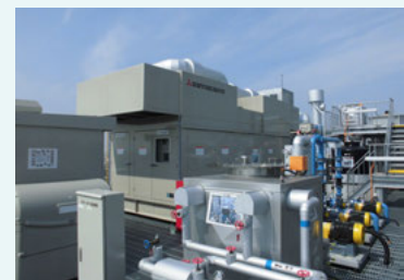
Newly introduced gas cogeneration system
