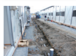
Plastic pipes KUBOTA's plastic pipes are being laid in projects to restore water supply systems and bring water to temporary housing, as well as to carry water out of flooded districts.
