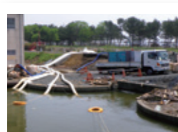
Drain pump vehicles Our drain pump vehicles are being deployed as needed for emergency water drainage and to combat flooding caused by heavy rainfall and spring tides.
