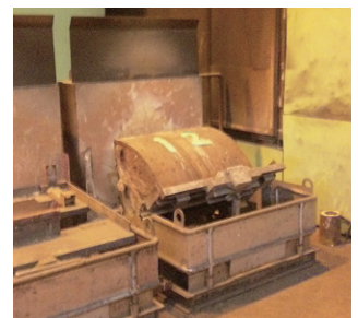
Ladle drying and preheating equipment
