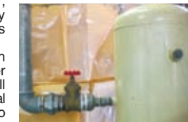
Enhancing energy efficiency by enlarging the diameters of air pipes
