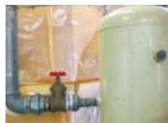
Enhancing energy efficiency by enlarging the diameters of air pipes
