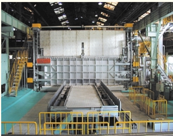
Entrance side for pipes
