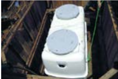
Small Johkasou in use for detached housing (Indonesia)
