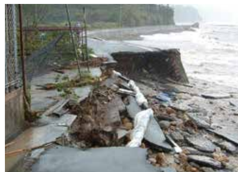
NS-type DN150 (6") after landslide
