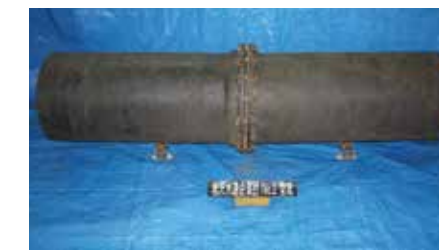
The pipes after 53 years in service
