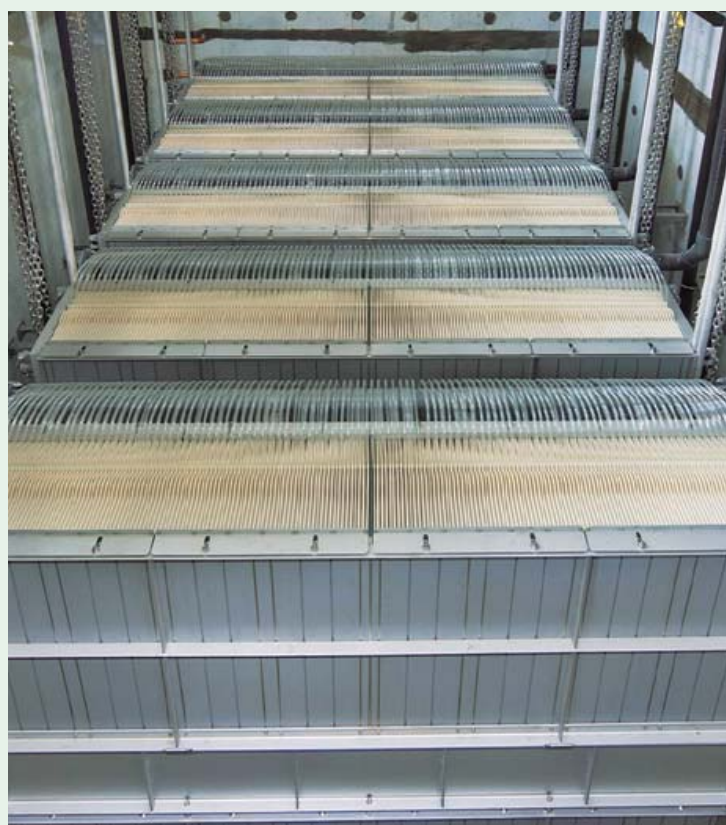
Submerged Membrane System
