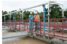
Constructed water treatment facilities in Myanmar
