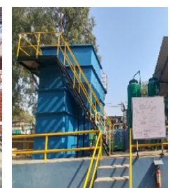
Sewage treatment plant (STP)
