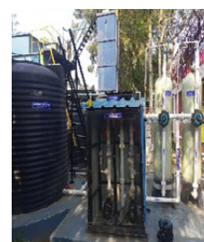
Equipment that allows the reuse of wastewater
