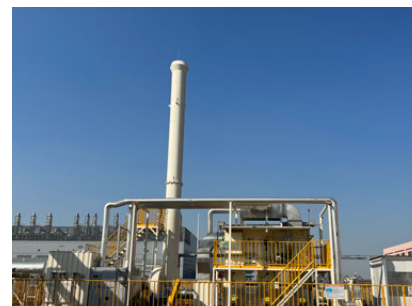
Kubota Engine (WUXI) Co., Ltd. (China) has installed a regenerative thermal oxidizer (RTO) and is working to reduce its VOC emissions.
