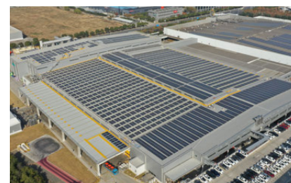
Solar power generation system installed on the rooftop of a plant in China
