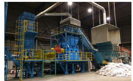
Plastic crushing and sorting facility
