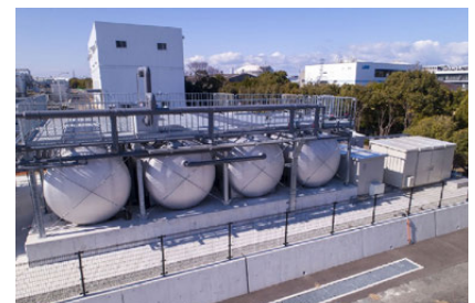
Kubota Sakai Rinkai Plant (Japan) Submerged-type FRP johkasou , decentralized wastewater treatment plants
