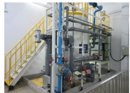
At Kubota Agricultural Machinery (Suzhou) Co., Ltd. (China), we installed recycling treatment equipment for reusing wastewater from processes throughout the entire plant, and this has realized zero emissions of process wastewater. In 2020, we reduced the amount of water usage by 140,000 m 3 .
