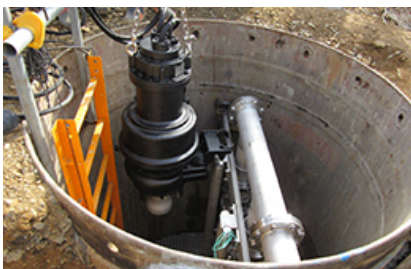
Manhole pumps (for pneumatic transportation of sewage)
