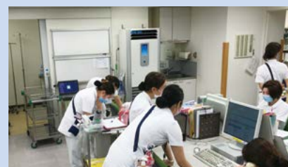
Installed in a nurse station
