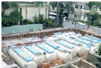
Large Johkasou in use at a hospital (Vietnam)
