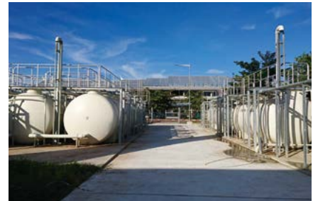
Johkasou: used to treat wastewater in areas where there are no sewage lines.
