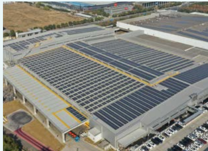
Solar panels installed
