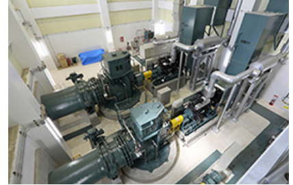
Pumps (used for emergency drainage as a countermeasure for flooding caused by heavy rainfall and high tides)
