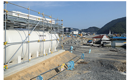
Wastewater treatment tanks (used to process wastewater from temporary housing in regions with insufficient sewage lines)
