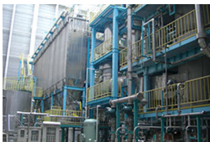
Water treatment plant (used to purify wastewater, including residential and industrial sewage)
