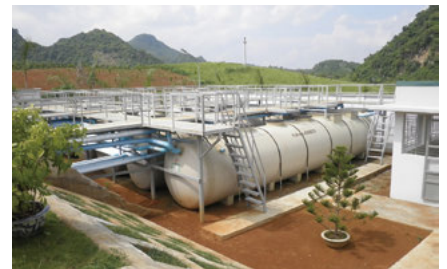
Wastewater treatment plants (Johkasou): used to treat wastewater in areas where there are no sewage lines.
