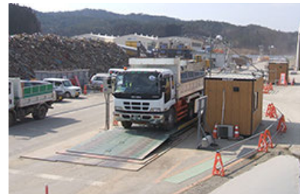
Truck scales (used to weigh truck cargo, such as debris)
