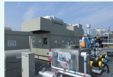
Newly introduced gas cogeneration system
