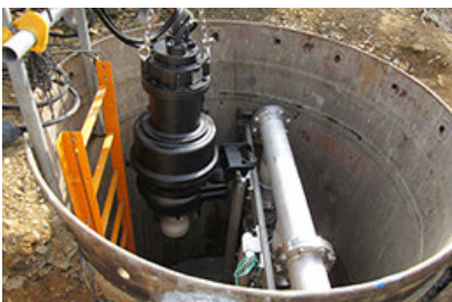
Manhole pumps (for pneumatic transportation of sewage)
