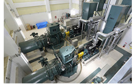
Pumps (used for emergency drainage as a countermeasure for flooding caused by heavy rainfall and high tides)
