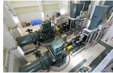
Pumps (used for emergency drainage as a countermeasure for flooding caused by heavy rainfall and high tides)
