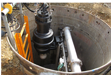
Manhole pumps (for pneumatic transportation of sewage)
