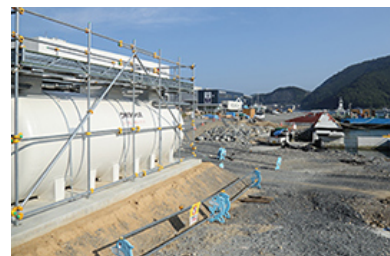
Wastewater treatment tanks (used to process wastewater from temporary housing in regions with insufficient sewage lines)
