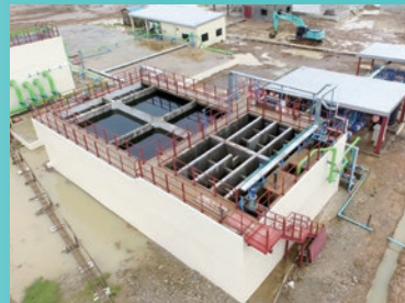
Water purification plant constructed in Thilawa Industrial Park Zone A
