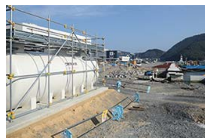
Wastewater treatment tanks This facility processes wastewater from temporary housing in regions with insufficient sewage lines.
