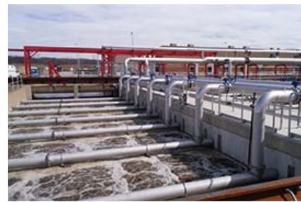
Kubota SMUs installed at the wastewater recycling facilities (top: before operation, bottom: in operation)
