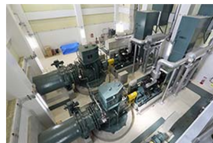
Pumps This is used for emergency drainage as a countermeasure for flooding caused by heavy rainfall and high tides.
