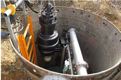
Manhole pumps (for pneumatic transportation of sewage)
