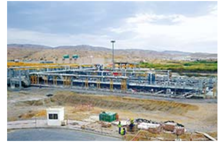
Al Ansab Sewage Treatment Plant (Oman)
