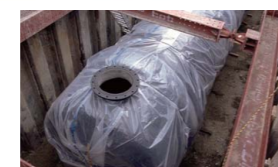
10 Earthquake resistant reservoirs: used to ensure the supply of drinking water when water services are halted due to an earthquake or other disaster.
