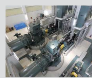
Pumps This is used for emergency drainage as a countermeasure for flooding caused by heavy rainfall and spring tides.
