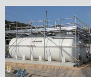
Waste water treatment tanks This facility processes wastewater from temporary housing in regions with insufficient sewage lines.
