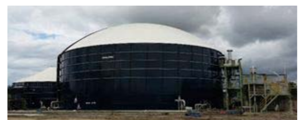
First palm oil mill effluent processing facility in Malaysia (for BBC Biogas) External view of membrane-type methane fermentation facility
