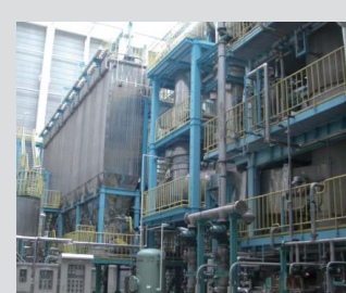
Water treatment plant This is used to purify waste water, including residential and industrial sewage.
