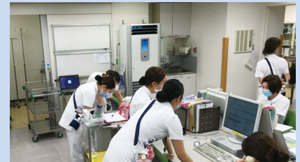
Installed in a nurse station
