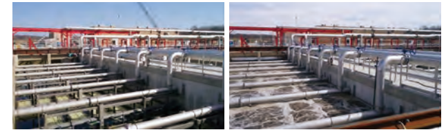
SMUs installed at the wastewater recycling facilities
