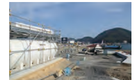
Wastewater treatment tanks
