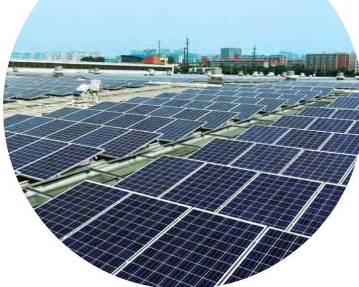
Solar panels installed at factory of Kubota Construction Machinery (WUXI) Co., Ltd
