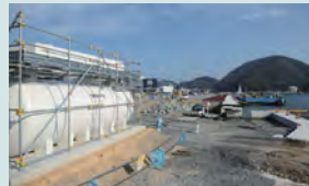
Wastewater treatment tanks
