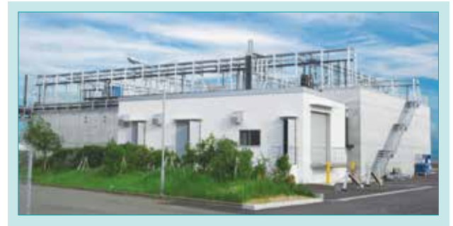
Fig. 3 Delivered Wastewater Treatment Equipment (Scale: 2500 m 3 /d)
