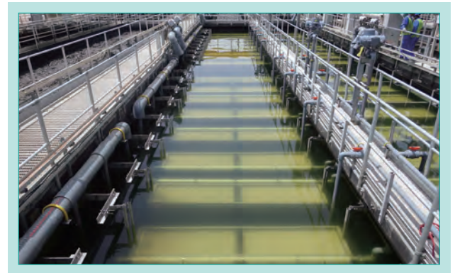
Fig. 8 Overview of Membrane Tank
