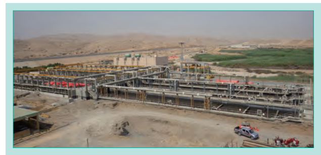
Fig. 2 Overview of MBR System
